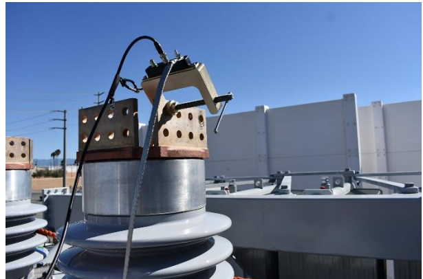
"Measure" lead connection to the large signal clamp
