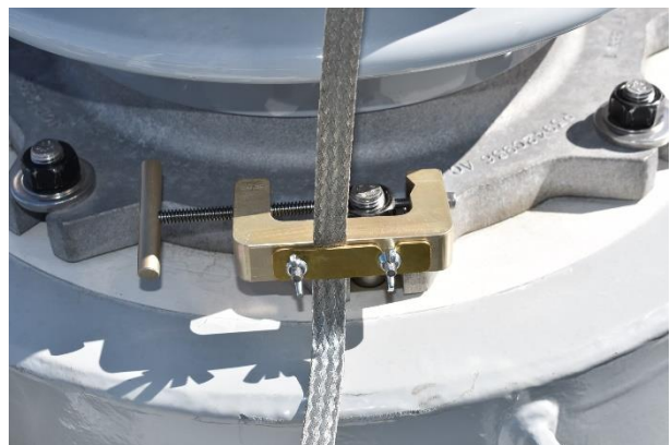
Earth connection to the ground clamp
